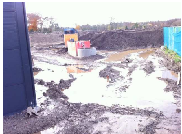
Waterlogged ground beside sales pod
