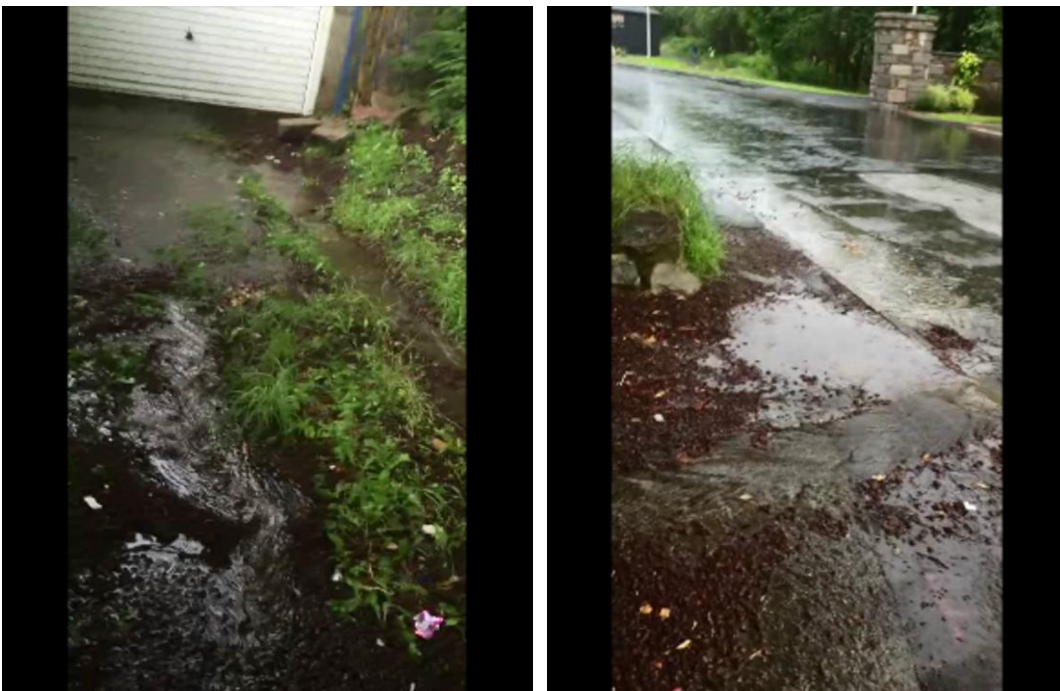
Flooding in the rear garden at NO.21 Pinewood Road
