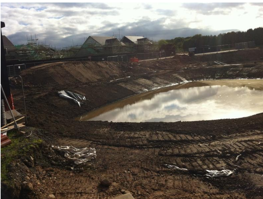
Outlet headwall from bottom retention pond – this pond is designed to always be full of water, the outlet is near the upper edge of the pond.
