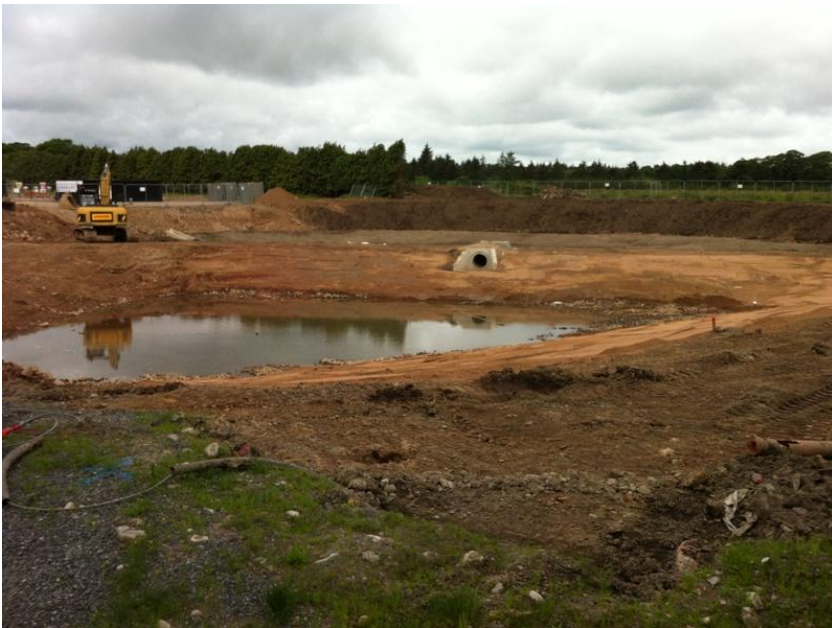
Outlet from Top pond to Bottom pond with 3.5m access path between two ponds
