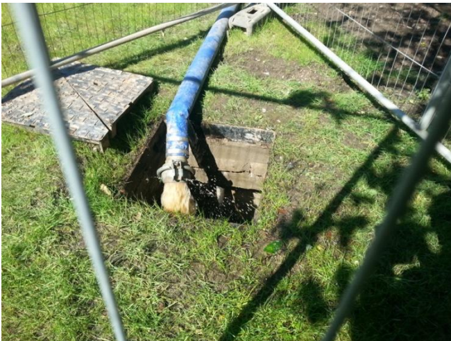
Water being pumped to a nearby drain
