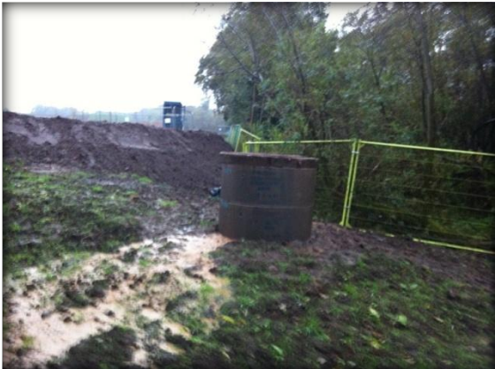
Water flowing out of concrete manhole at the bottom of the site near burn
