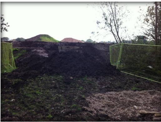
Dandara built soil up around the concrete manhole to try and stop water leaking out and running down the footpath or into the burn.
