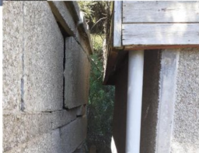
Photo 9 – Viewed from neighbours property. Displacement of boundary wall.
