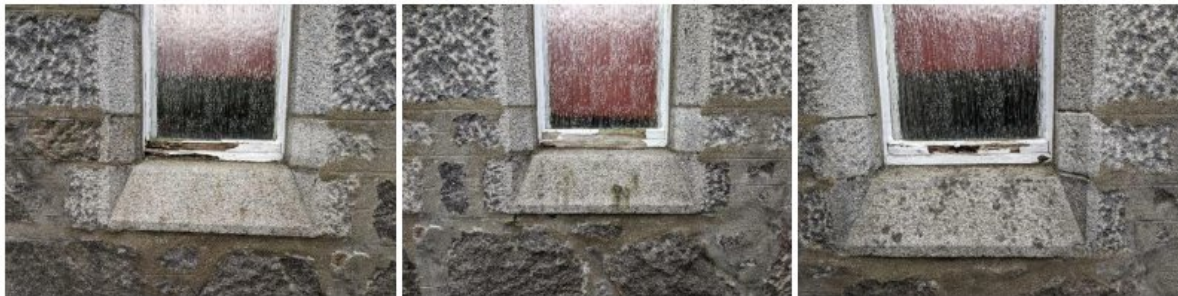
Images of the rotten window frames
