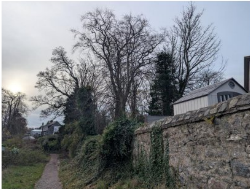
Photo 5 – Large, mature beech 4787 and sycamores 4789 and 4790 require to be pruned due to their proximity to neighbouring properties. The trees are exposed by the failure and removal of adjacent trees.
